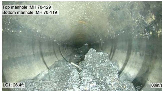
Obstruction Rocks from 3 to 9 o'clock, Loss of cross sectional area = 30% After Heavy Cleaning Debris Still Exist In Pipe
