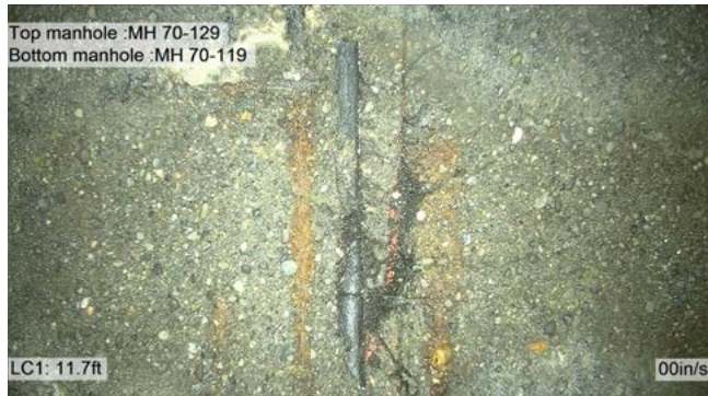
Hole from 10 to 3 o'clock, Length = 6 in., Joint, Exposed Sealing Gasket
