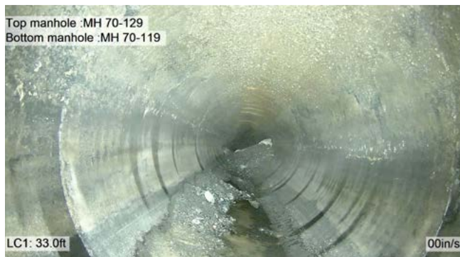
Miscellaneous Water Level Sag, Water Level = 50%, Continuous Water Sag
